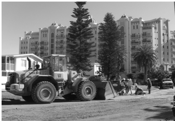
Workers lay the new water main in the first phase of our streetscape program. Sanitary and storm sewers will be next.
